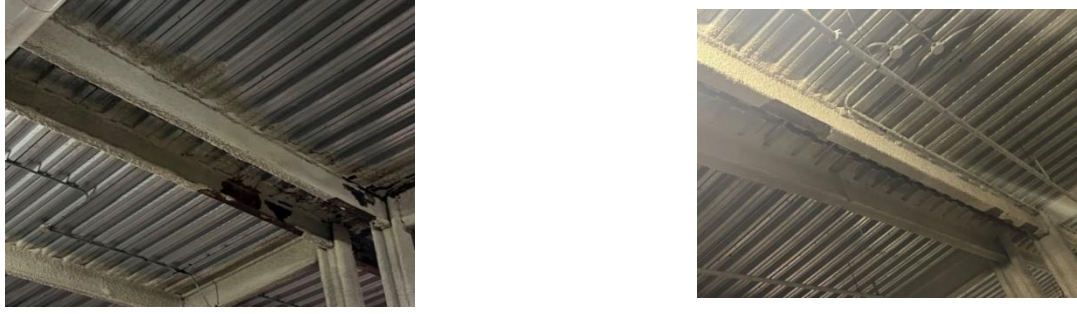
Figure 2 Illustration of defective SFRM on primary beam on the 1 st floor of a high-rise residential building.
